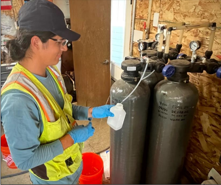
Tanaq-Sundance contractor Willem Martin takes a water sample from a Point of Entry Treatment system in East Selah as part of the Army's continued performance monitoring of the treatment systems.
