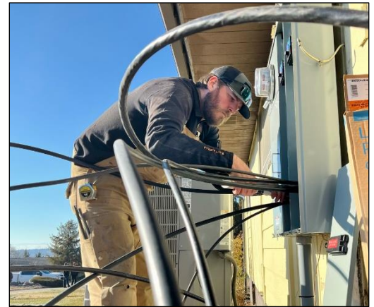
Wild West Electric LLC contractor Zack Briscoe installs a new electrical service box at an East Selah home to bring it up to code before power can be provided to a Point of Entry Treatment system.
