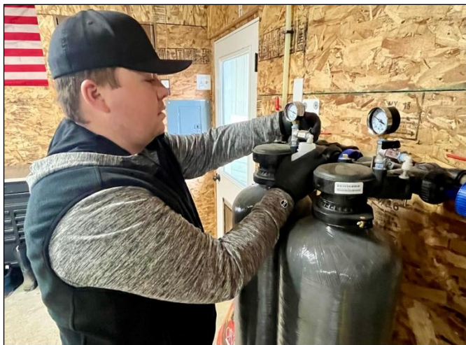
An Army contractor samples water from a Point of Entry Treatment system, which are effectively removing PFAS from the water in the East Selah area.
