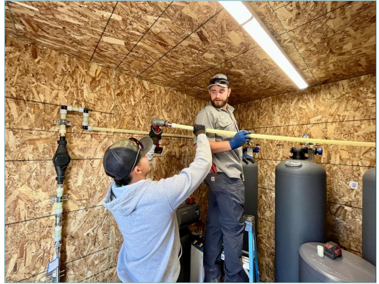
Army contractors install a Point of Entry Treatment (POET) system in a shed at an East Selah home. The Army is installing POET systems to remove PFAS from the water entering the home.
