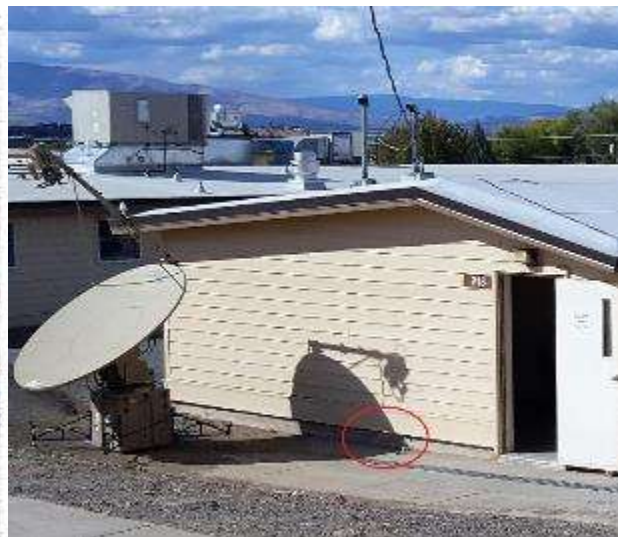
Figure 2-2: Grounding Rod – TCN
