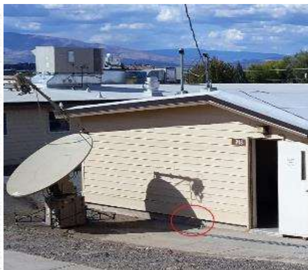
Figure 2-2: Grounding Rod – TCN
