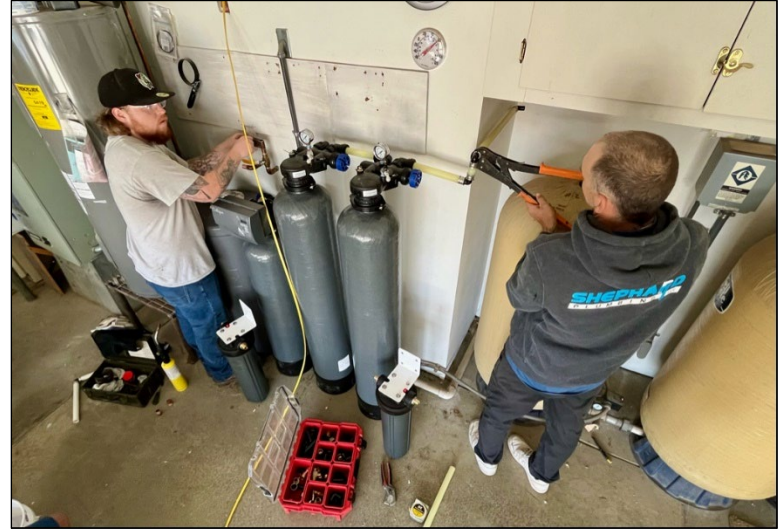
Army contractors install a Point of Entry Treatment (POET) system in the garage of an East Selah home. The Army is installing POET systems in homes where PFAS levels are at or above 70 ppt.
