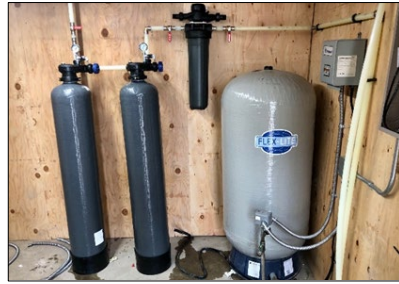
(Left and Below) This POET installation was split between an existing pump house and the homeowner's garage. Each system is designed specifically for each home.
