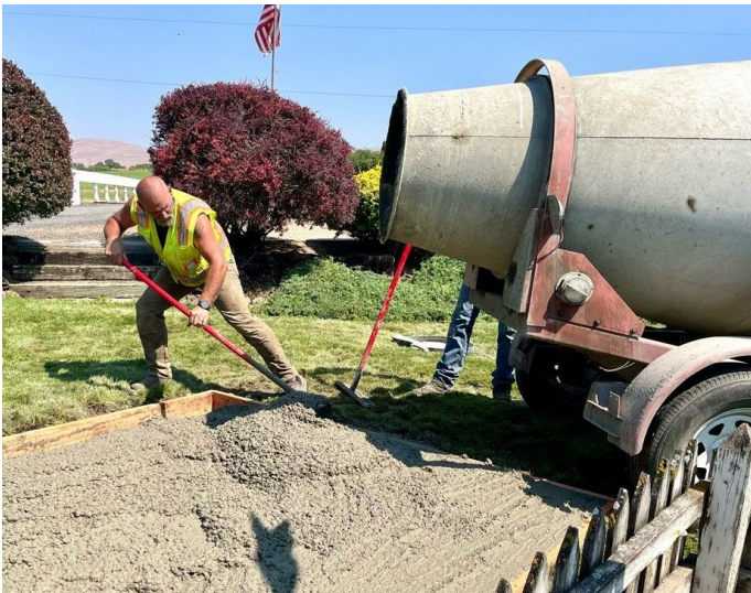
An Army subcontractor spreads concrete to form an 8-by-10-foot slab floor of a Point of Entry Treatment (POET) system shed at a home in the East Selah community. The Army is installing POET systems to remove PFAS from the water entering the home.
