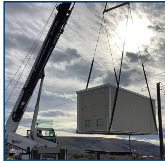
Delivery of the first residential Group B POET system enclosure.
