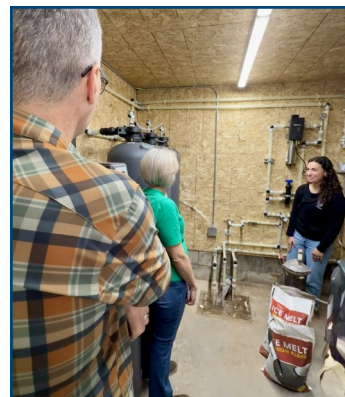
Army contractor, ECC, gives a tour of a residential POET system to DoW representatives.
