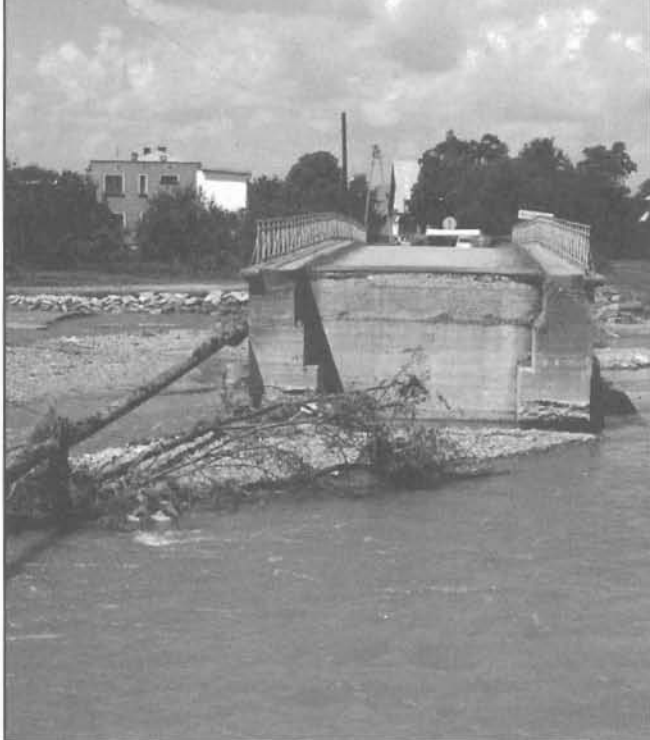
Figure 2. A washed out embankment behind a bridgehead. A 60-meter section of the access road was destroyed (Bystrzyca Dolna town - Bystrzyca River).
