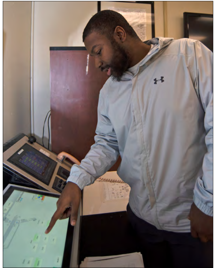
Ronald Williams, an airfield operations specialist intern, checks the lighting control panel to ensure the flightline lights are on. During inclement weather, the lights on the runway remain on for visibility.
