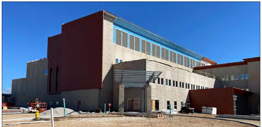
A view of the emergency department entrance. All of the facilities' exterior components are nearing completion.
