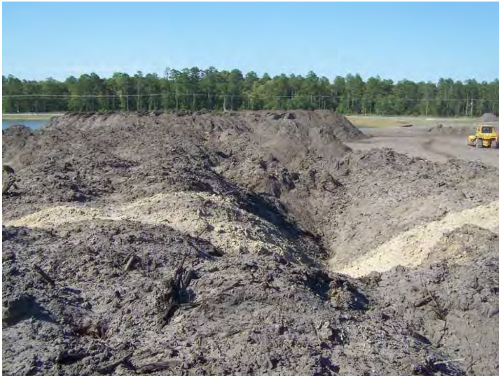
Inspected soil piles on the west side of the South Pond site
