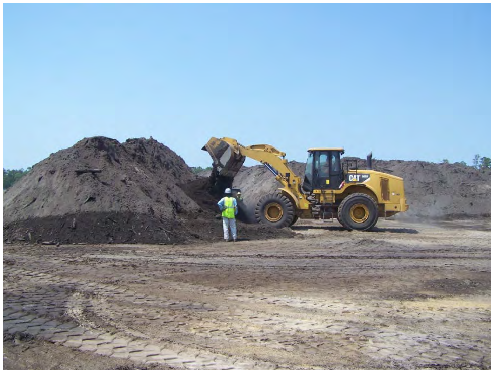
Working soil pile at the west side of the South Pond site
