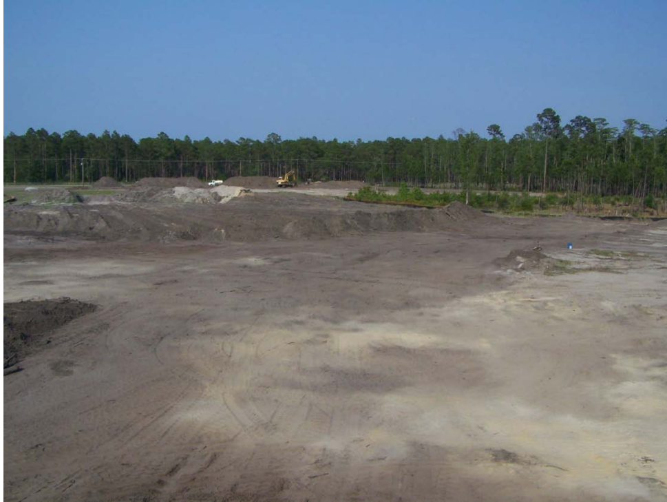
The current progress at the west side of the South Pond site
