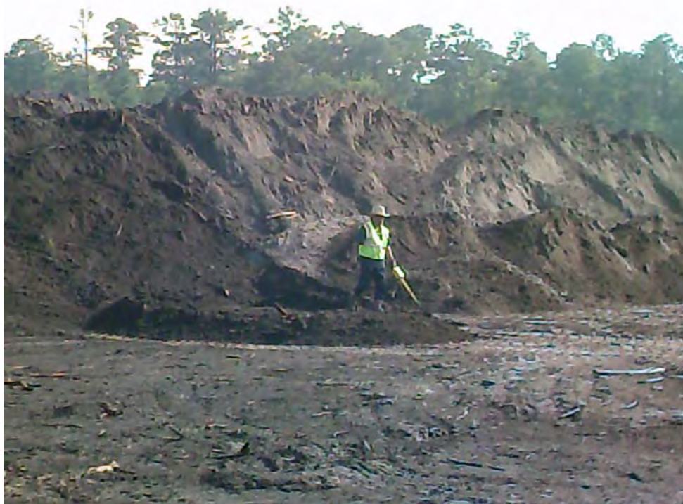
QC inspection of every 3 rd bucket at the west side of the South Pond site
