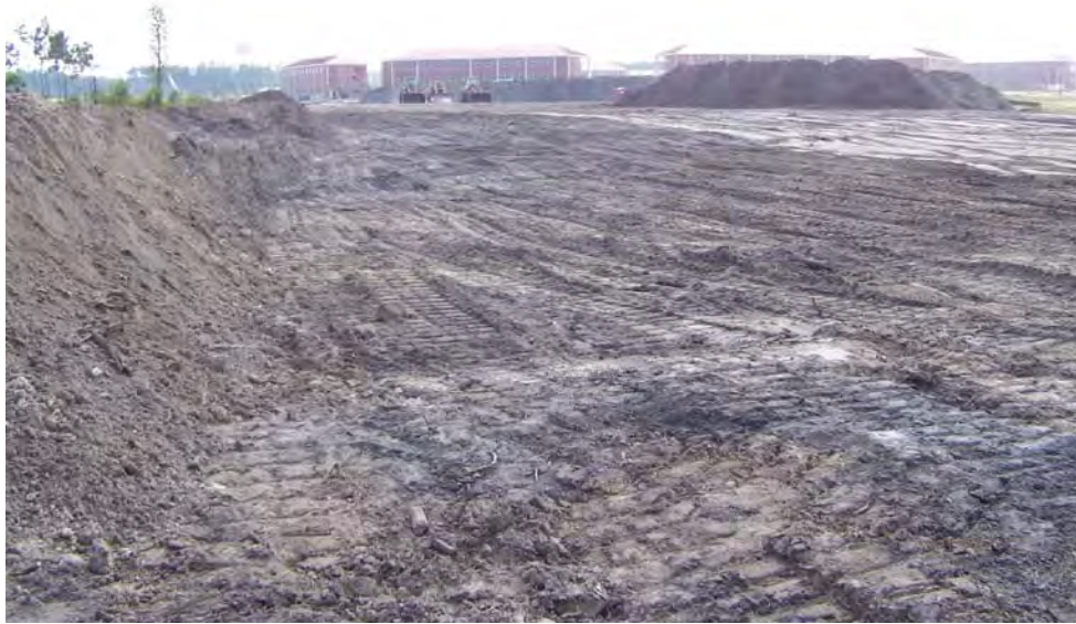
West side of the South Pond site possibly cleared to grade (awaiting surveyor conformation)
