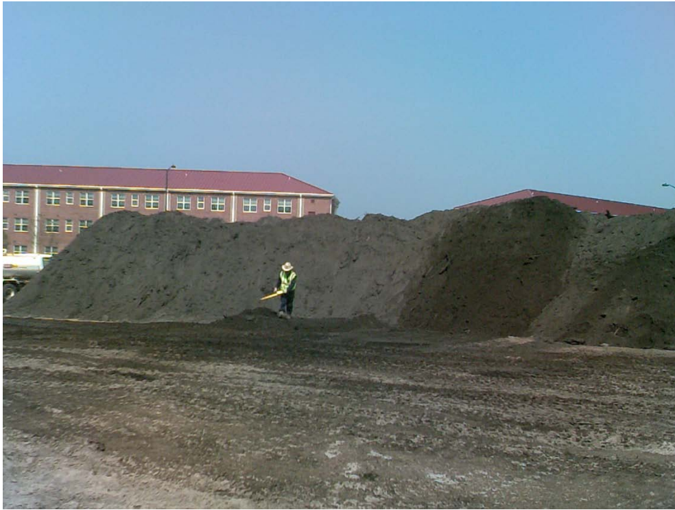
QC inspection of soil piles at the west side of the South Pond site
