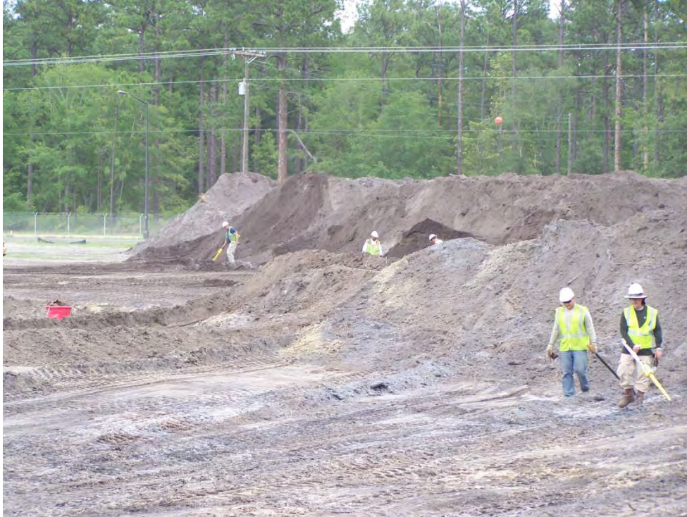
Working the soil pile on the east side of the South Pond site
