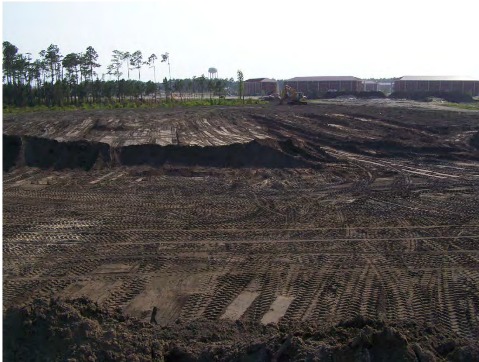
The current progress at the east side of the South Pond site
