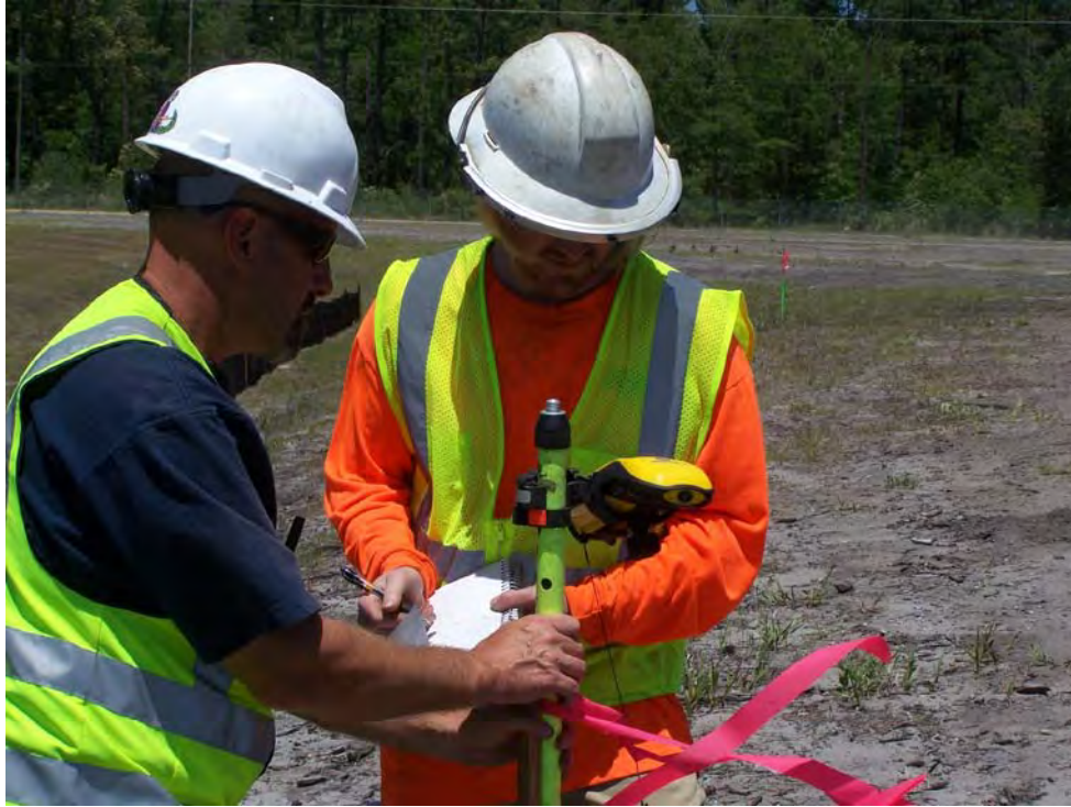
Plotting QC area on the east side of the South Pond site for clean soil placement
