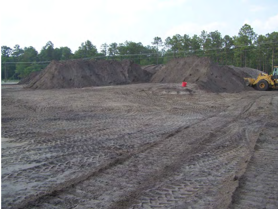
Clean spoils pile at the east side of the South Pond site
