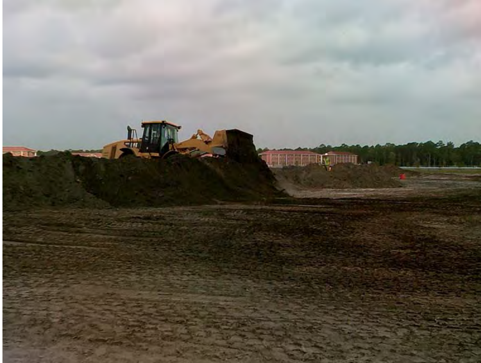
966H Front end loader working soil at the east side of the South Pond site
