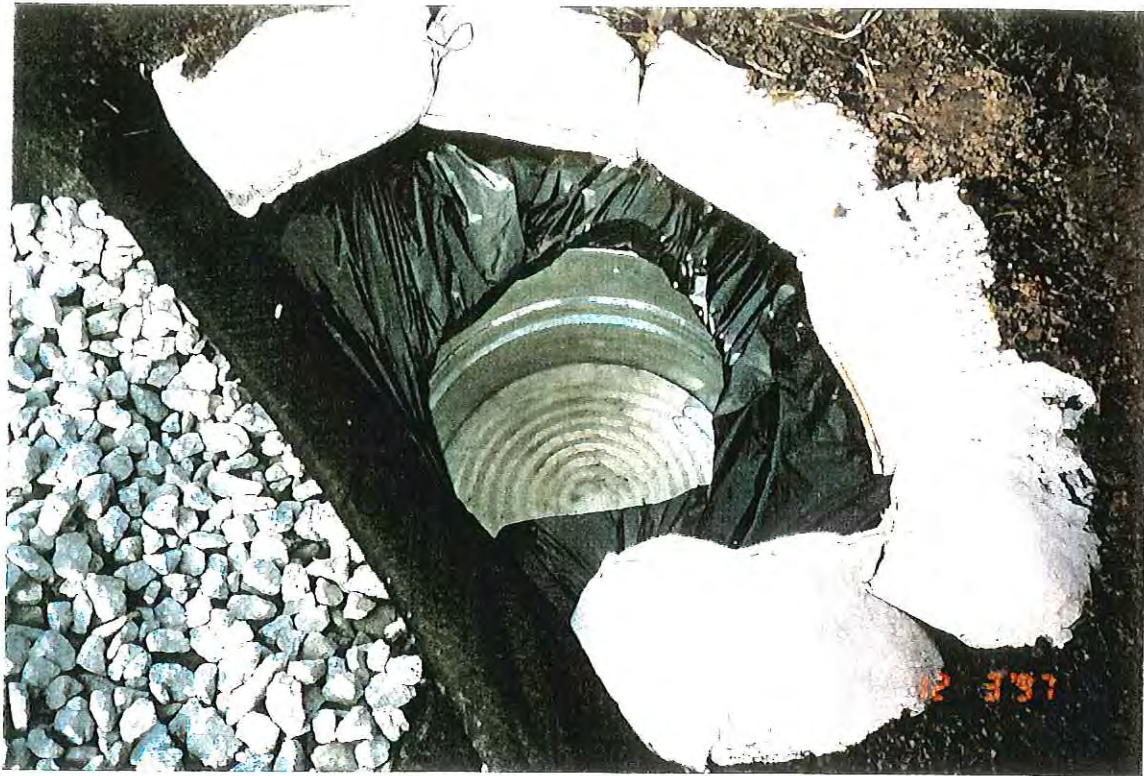
PHOTOGRAPH -35- DECON PAD SUMP
