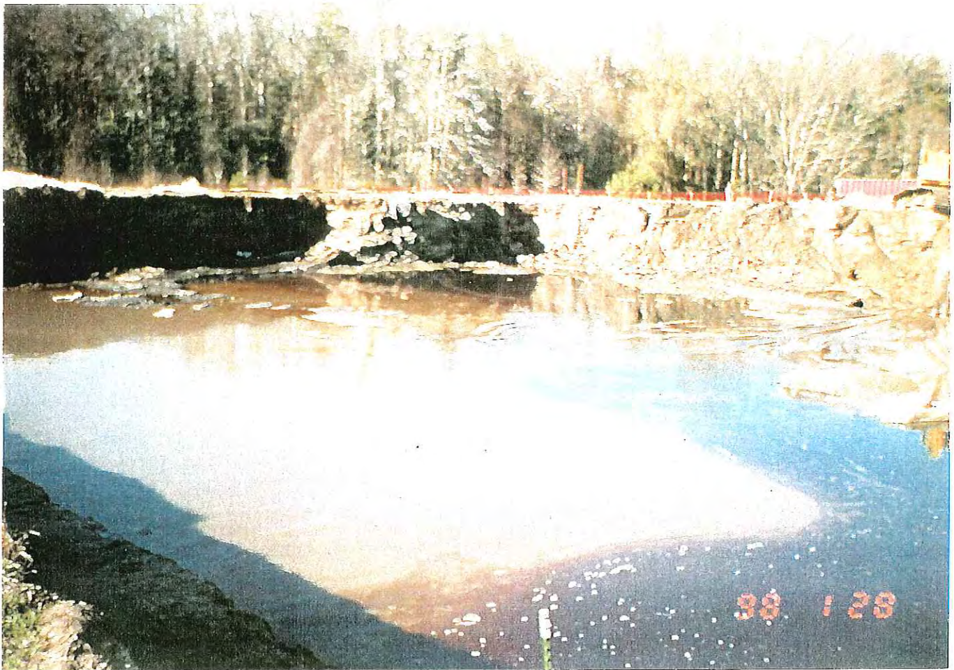
PHOTOGRAPH -67- FREE PRODUCT IN EXCAVATION
