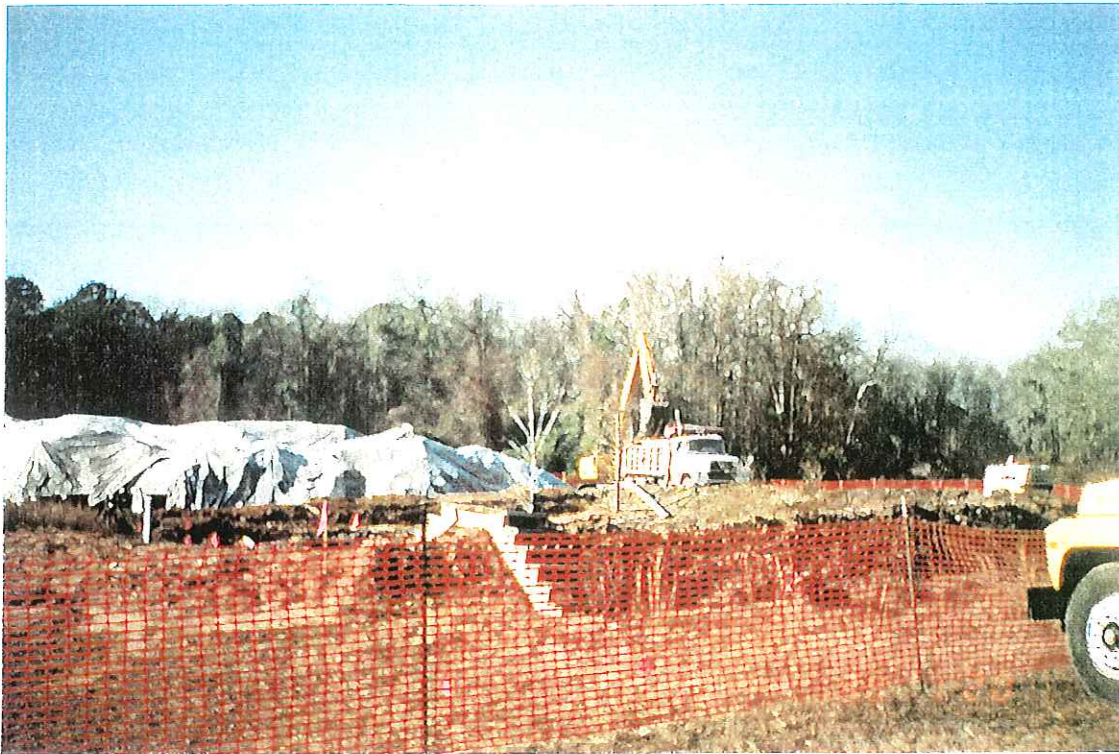
PHOTOGRAPH -65- COVERED STOCKPILED SOILS
