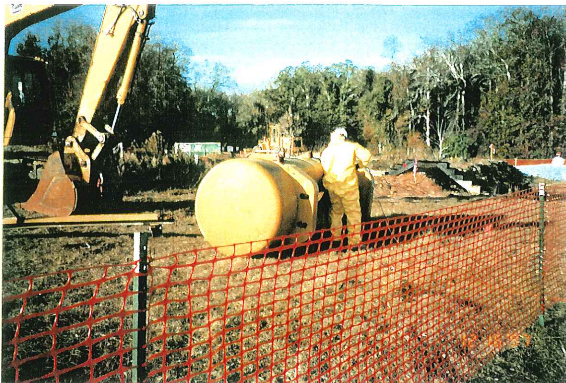
PHOTOGRAPH -45- 1100 GALLON ALUMINUM TANK
