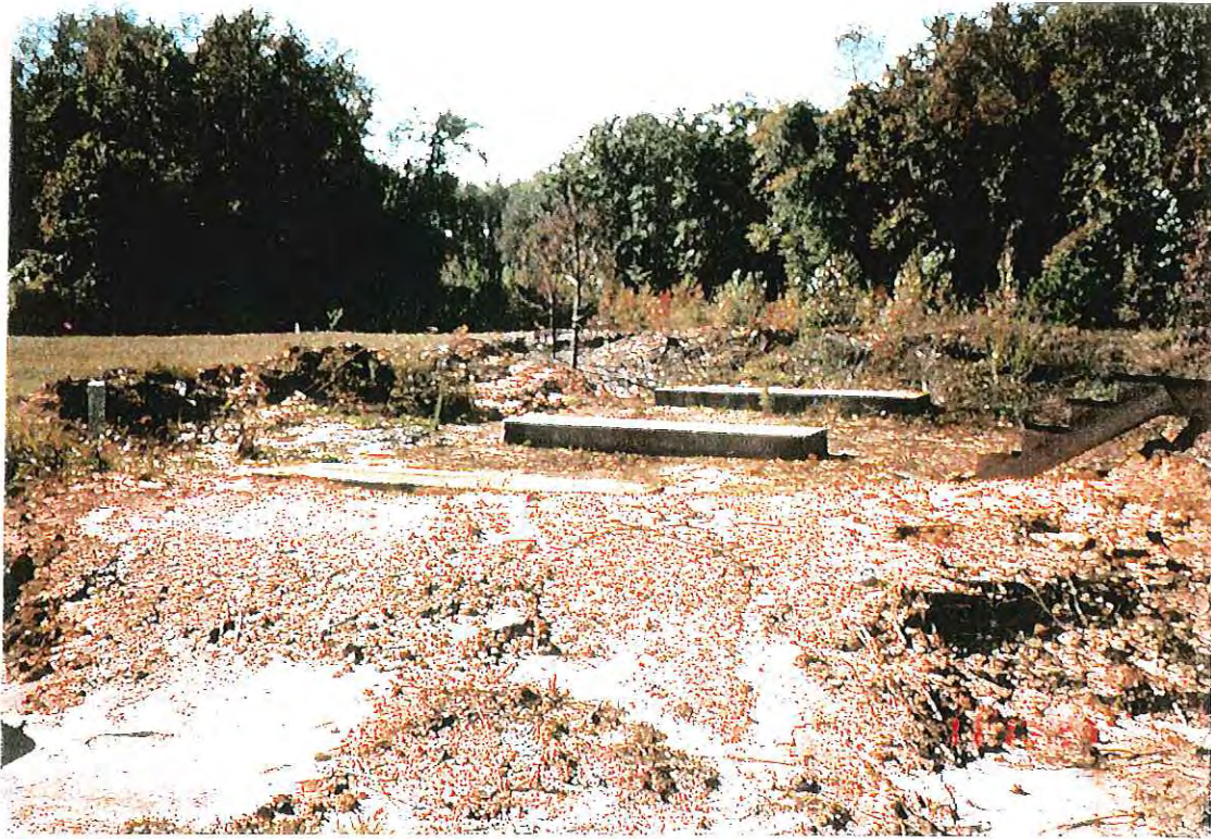
PHOTOGRAPH -15- CONCRETE CRADLE SUPPORTS FOR 17,000 GALLON AST
