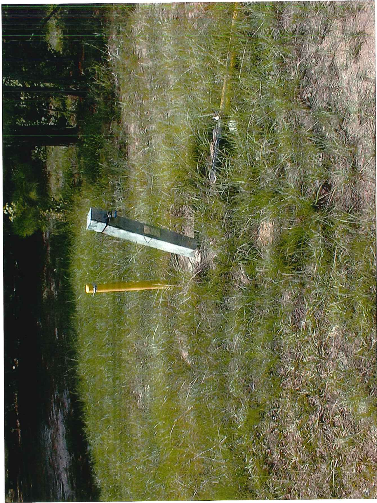
SWMU13: Monitoring Well 1
