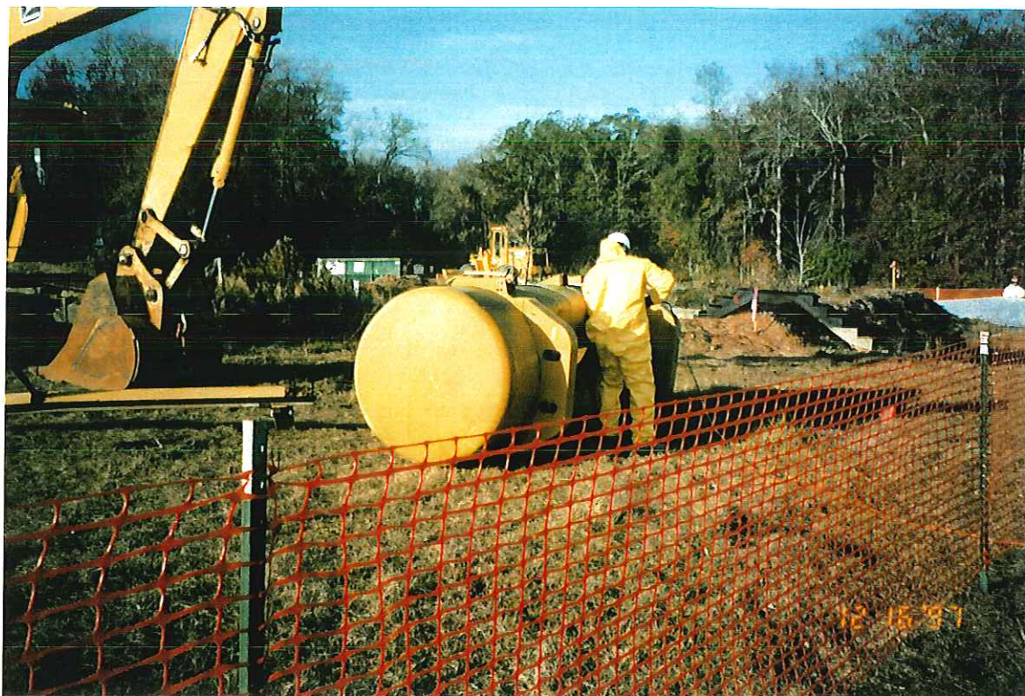
PHOTOGRAPH -45- 1100 GALLON ALUMINUM TANK
