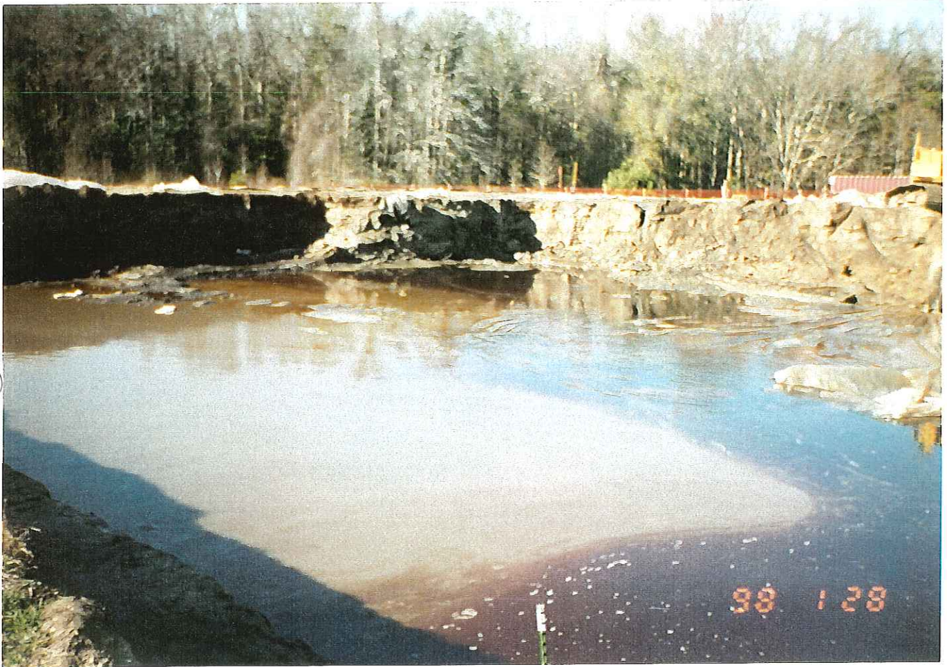
PHOTOGRAPH -67- FREE PRODUCT IN EXCAVATION
