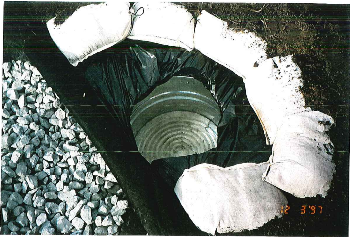
PHOTOGRAPH -35- DECON PAD SUMP
