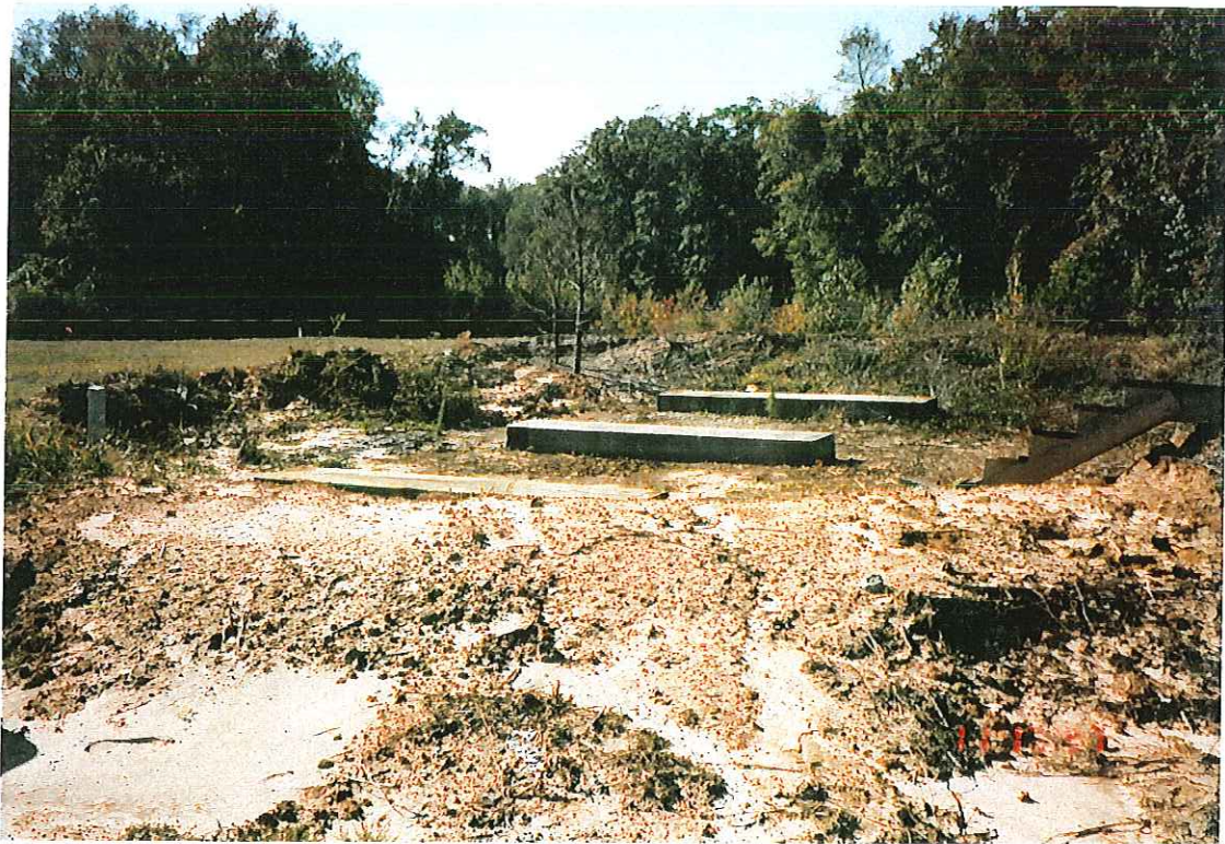
PHOTOGRAPH -15- CONCRETE CRADLE SUPPORTS FOR 17,000 GALLON AST
