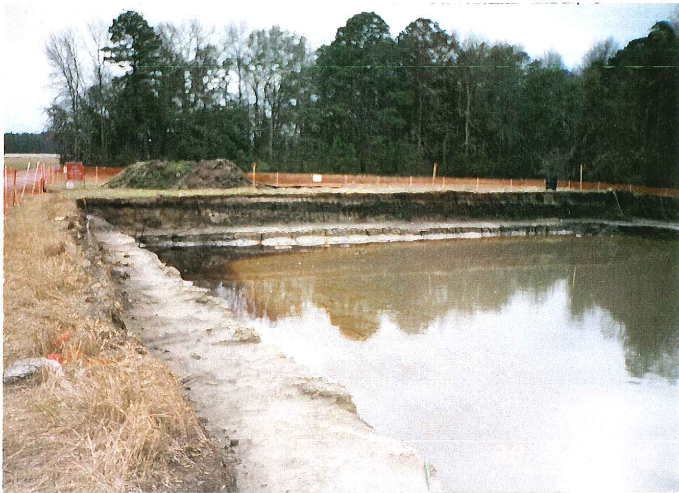
PHOTOGRAPH -79- FREE PRODUCT IN EXCAVATION
