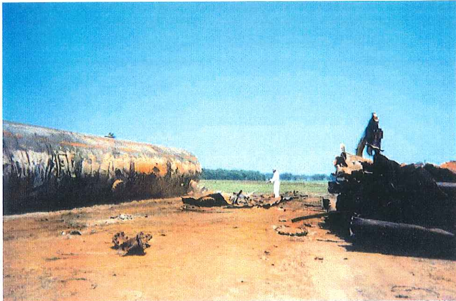
Pumphouse #6: Rinsing Tank #91.
