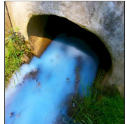
Illicit Discharge, Prince William County, Virginia
