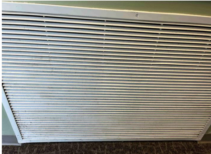
Figure 3: Dusty HVAC Return Vent
