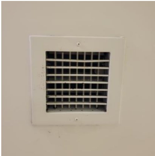
Figure 2: Dusty Bathroom Return Vent
