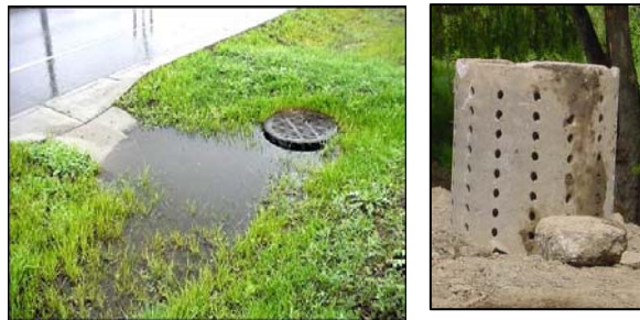
Typical UIC stormwater wells (drywells)
