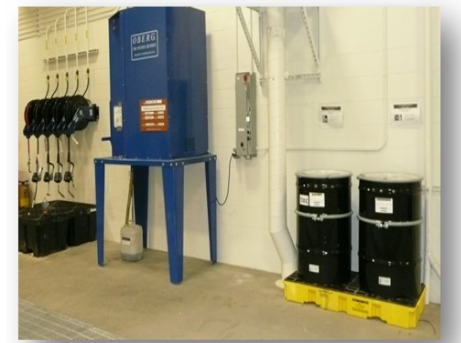
Unit Hazardous Waste Satellite Accumulation Areas
