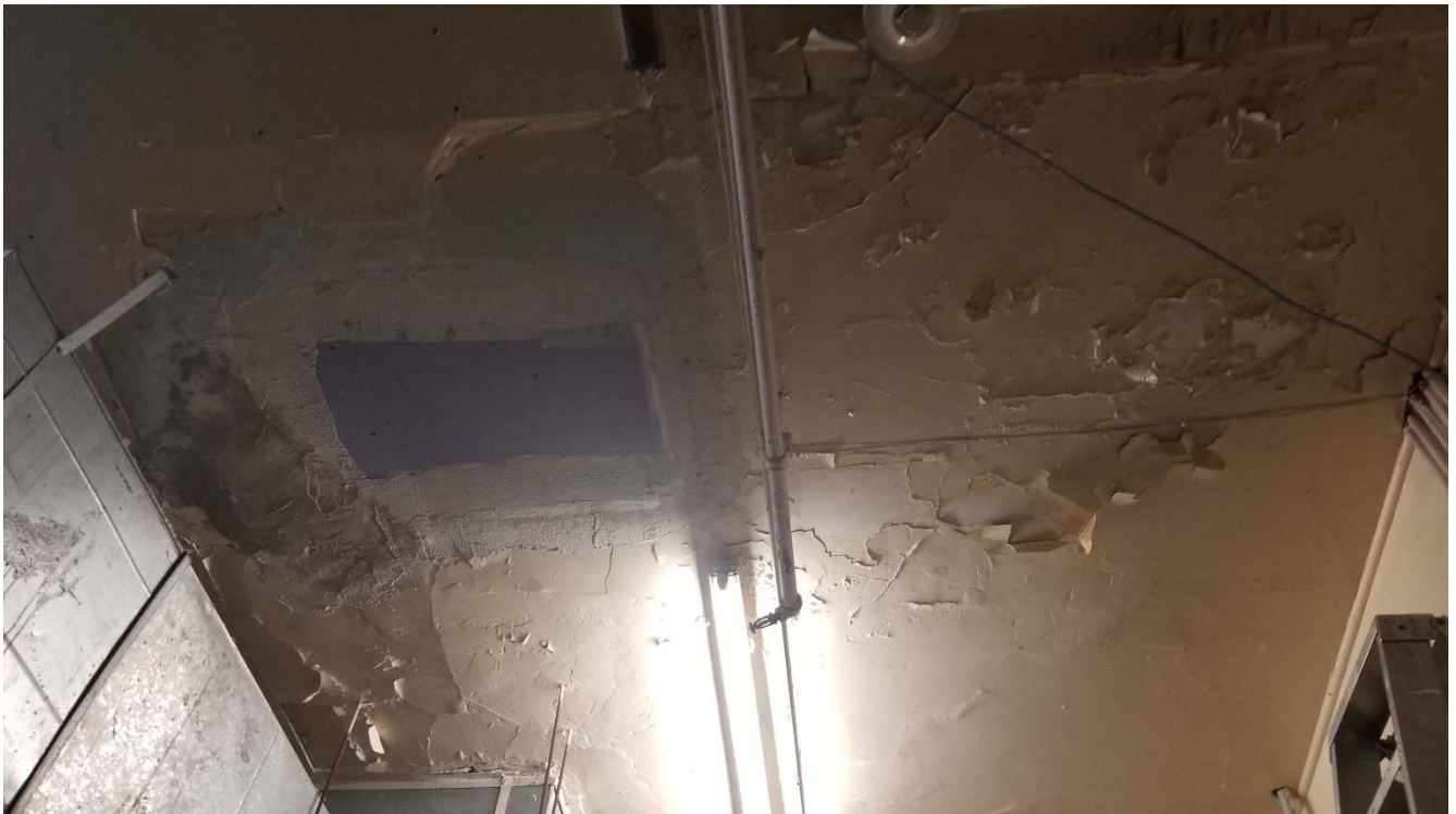
Ceiling water damage
