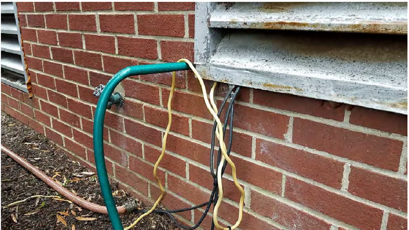
Bathhouse HVAC Louver – Possible Point of Entry for Rodents
