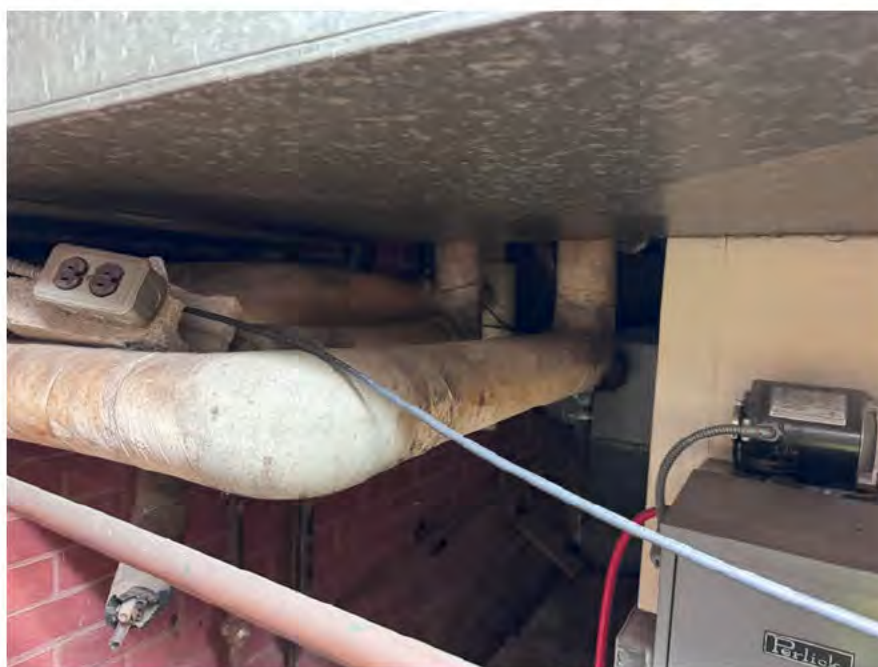
Photo 2: White mastic on TSI in Mech. Room 034 (Sample #2).
