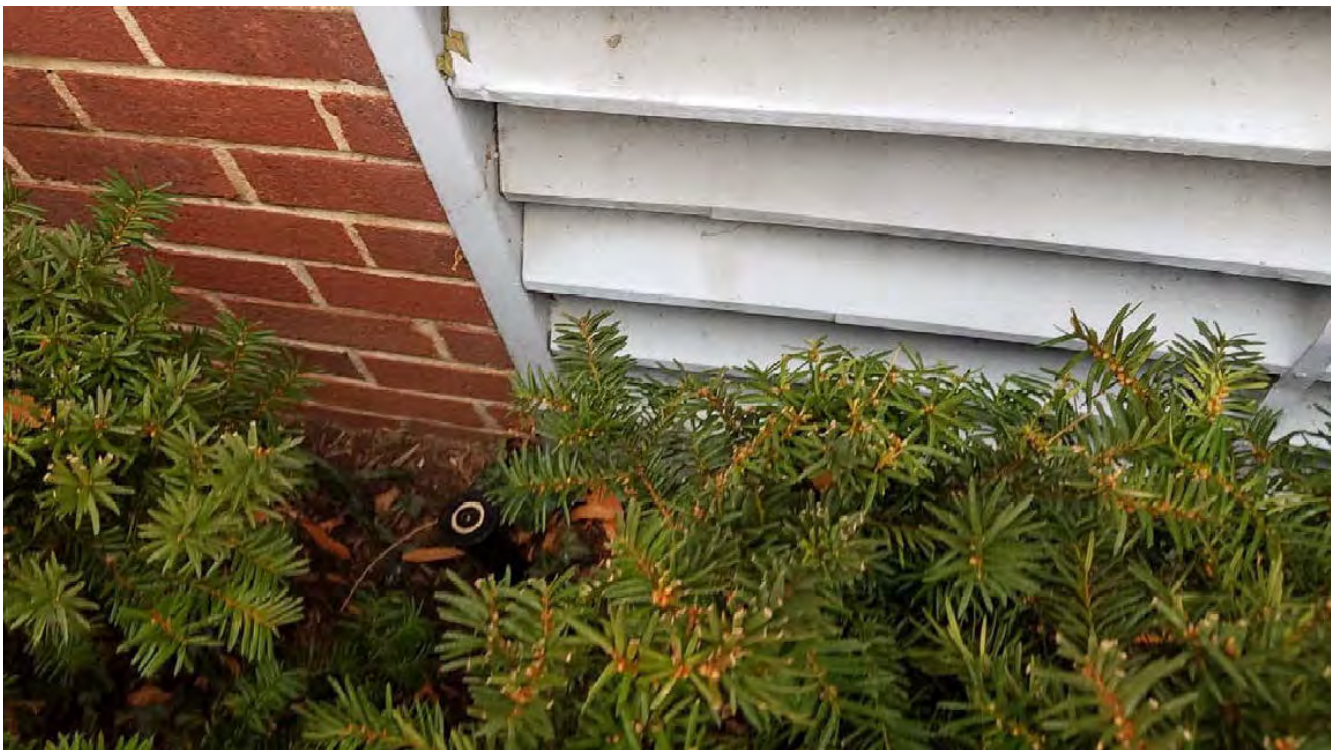
Outside Air Intake at Grade with Irrigation Head in Front of It
