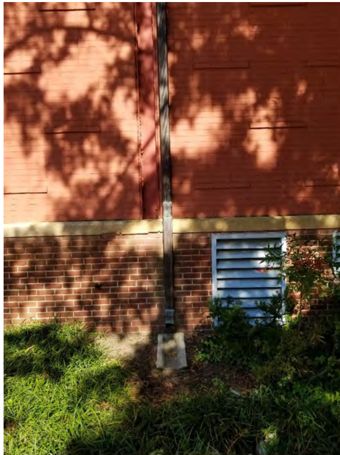
Air intake at grade adjacent to downspout
