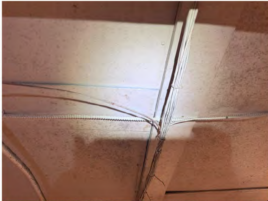
Photo 7: ACM Transite panel observed on the ceiling of Basement Mech. Room 006 (Sample #50).
