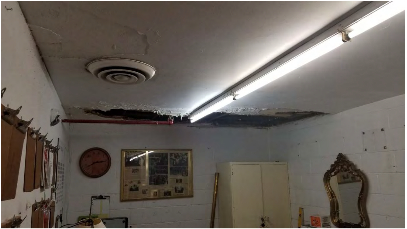
Water damaged ceiling
