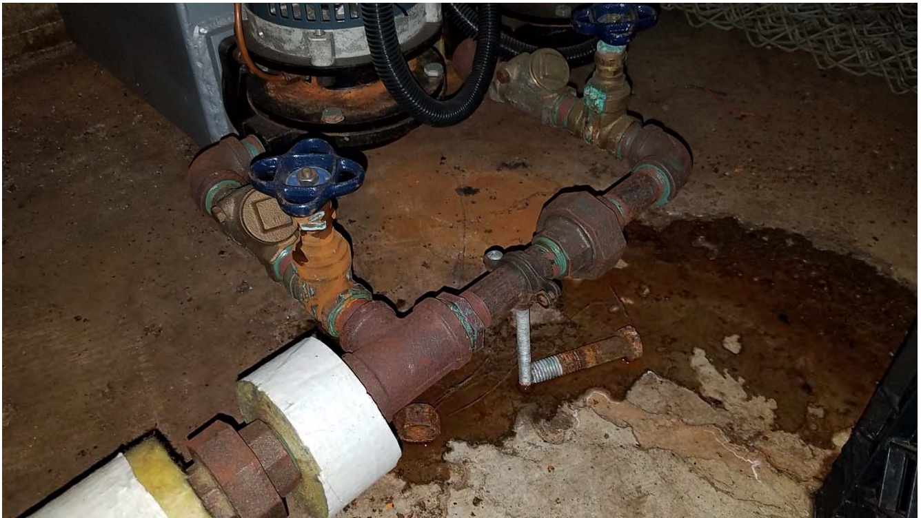
AHU-5 Low Pressure Condensate Lift Station Leaking
