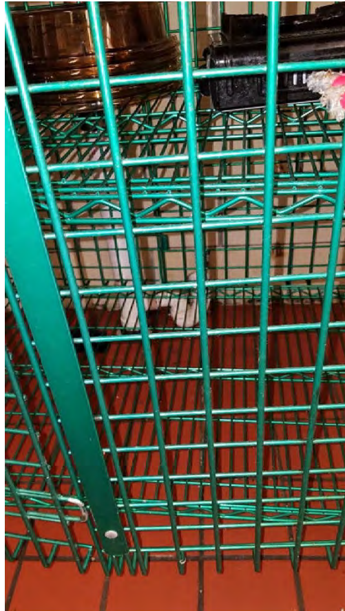
Open Hub P-Trap in Second Floor Kitchen
