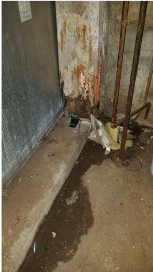
Standing water in mech room
