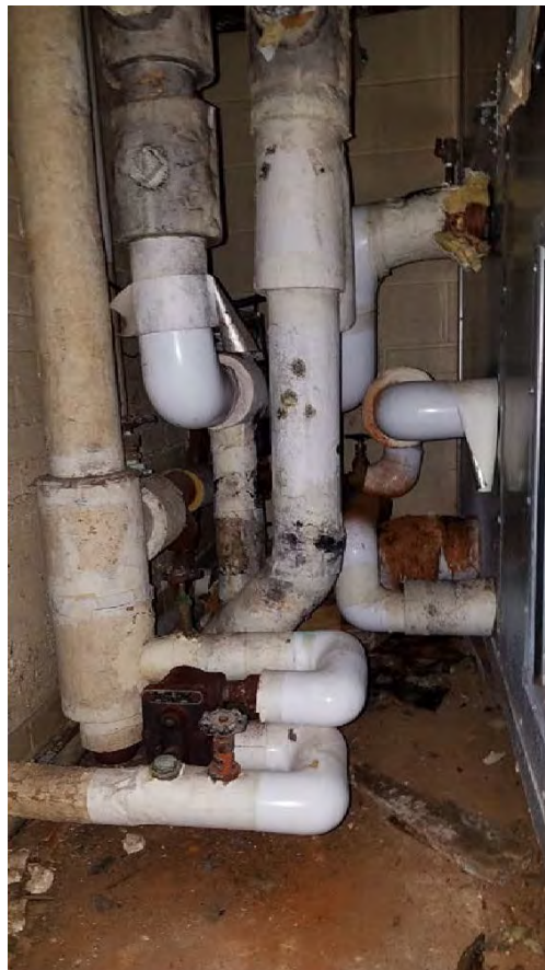
Bathroom AHU Pipe Chase and Mixed Air Plenum
