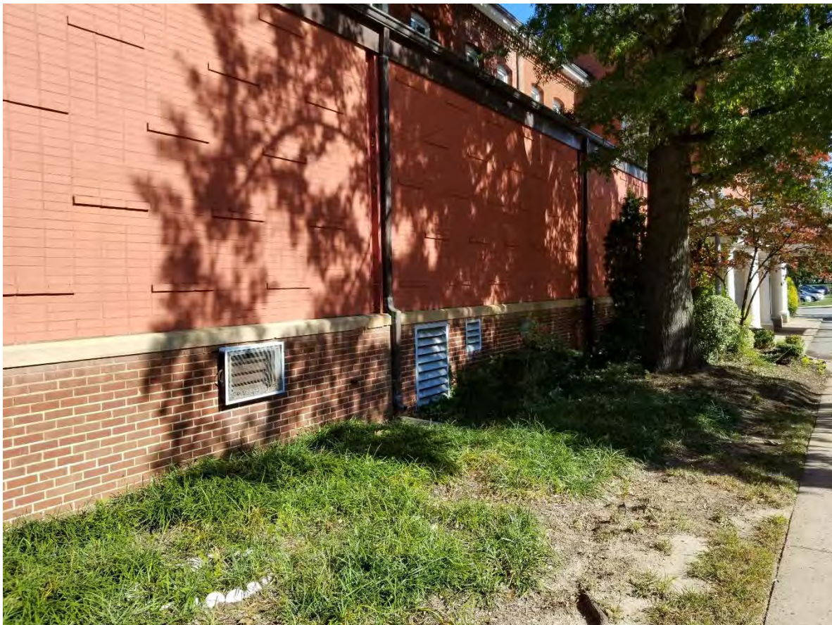
Low air intakes
