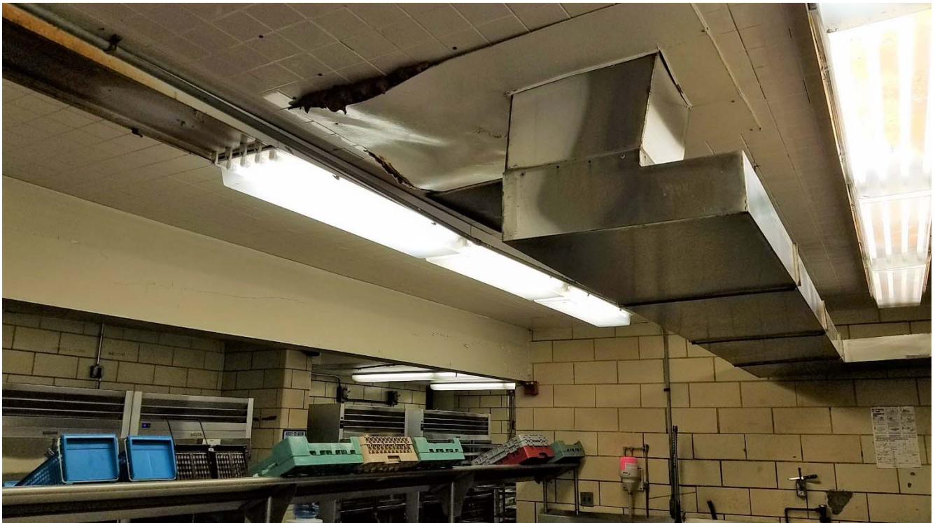
Moisture Laden Insulation at Duct Penetration in Second Floor Kitchen Dishwashing Area
