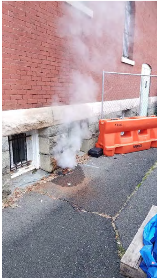
Mechanical Room 1 LPC Lift Station Vent
