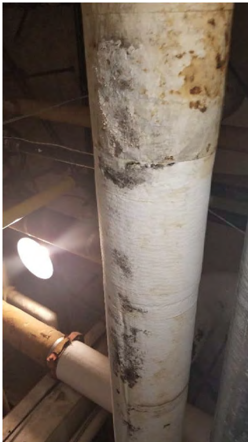
Mold on fiberglass pipe insulation
