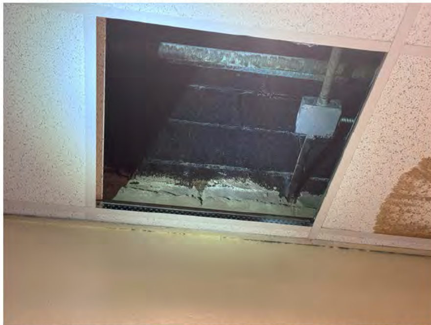
Photo 14: ACM black mastic observed on the CMU wall above the SACT in Kitchen Corridor 129 (Sample #132 & #133).
