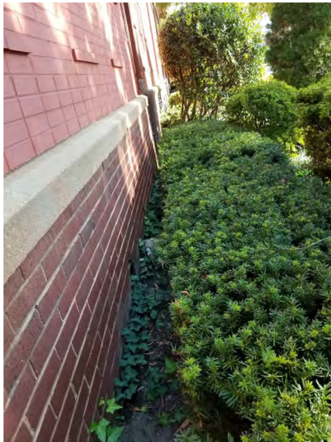
Hedges blocking access to roof drains
