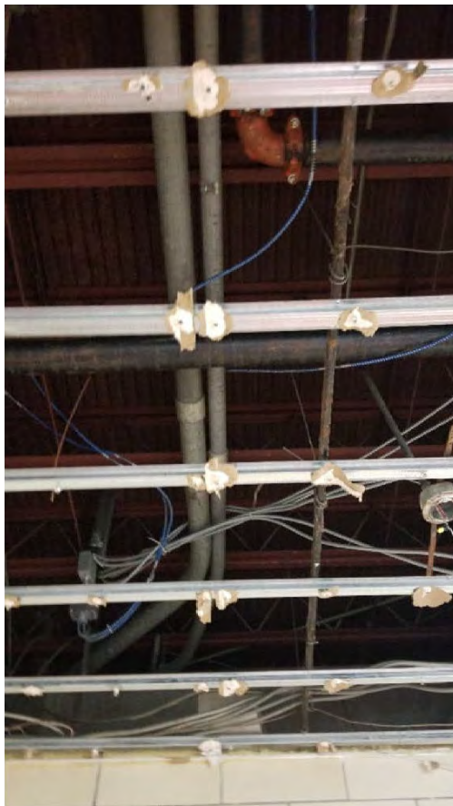
Ceiling water damage
