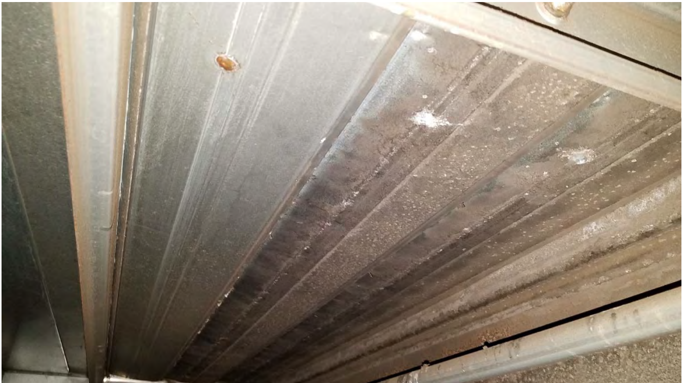
AHU-5 OA Damper in the Closed Position During Occupied Hours
