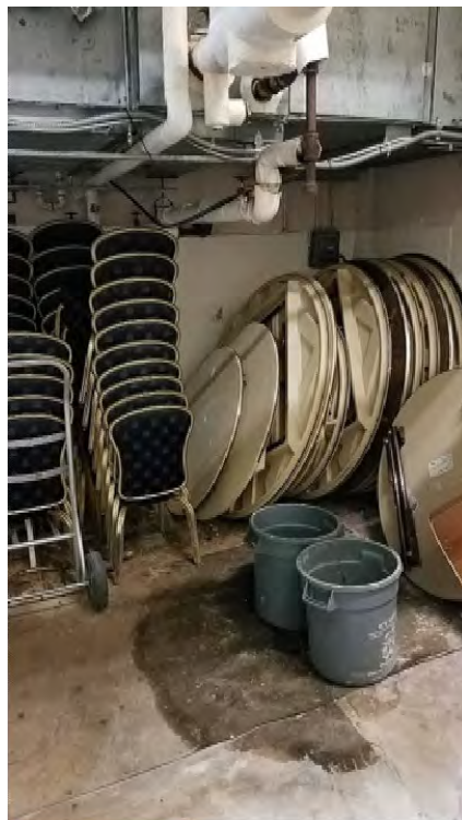
Leaking Low Pressure Condensate Pipe Contributing to Mold Garden in Coat Check Mechanical Room
