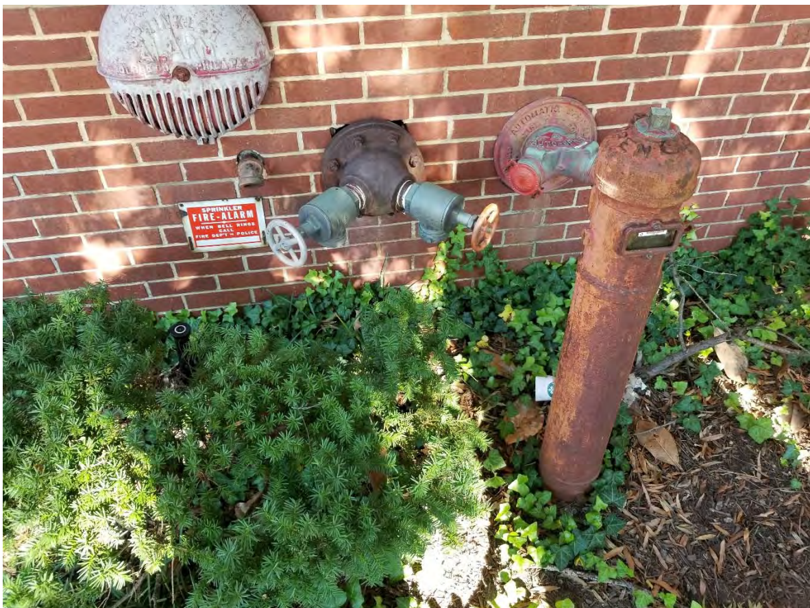
Irrigation spout in hedges at grade near facility
