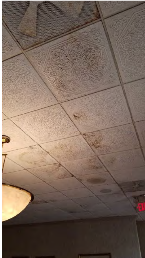
Ceiling water damage
