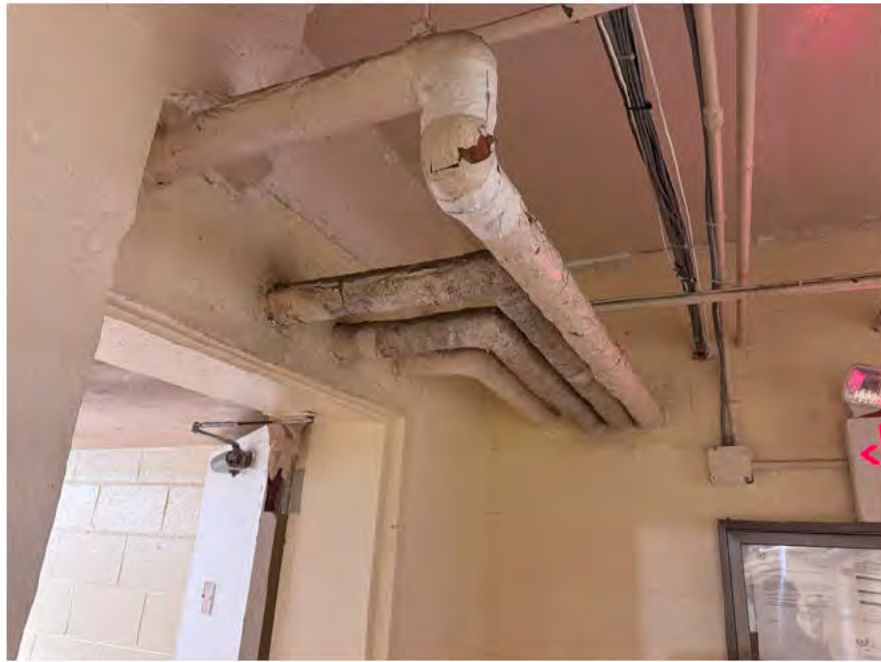
Photo 27: ACM mudded pipe fittings observed in Basement Vestibule 039.
