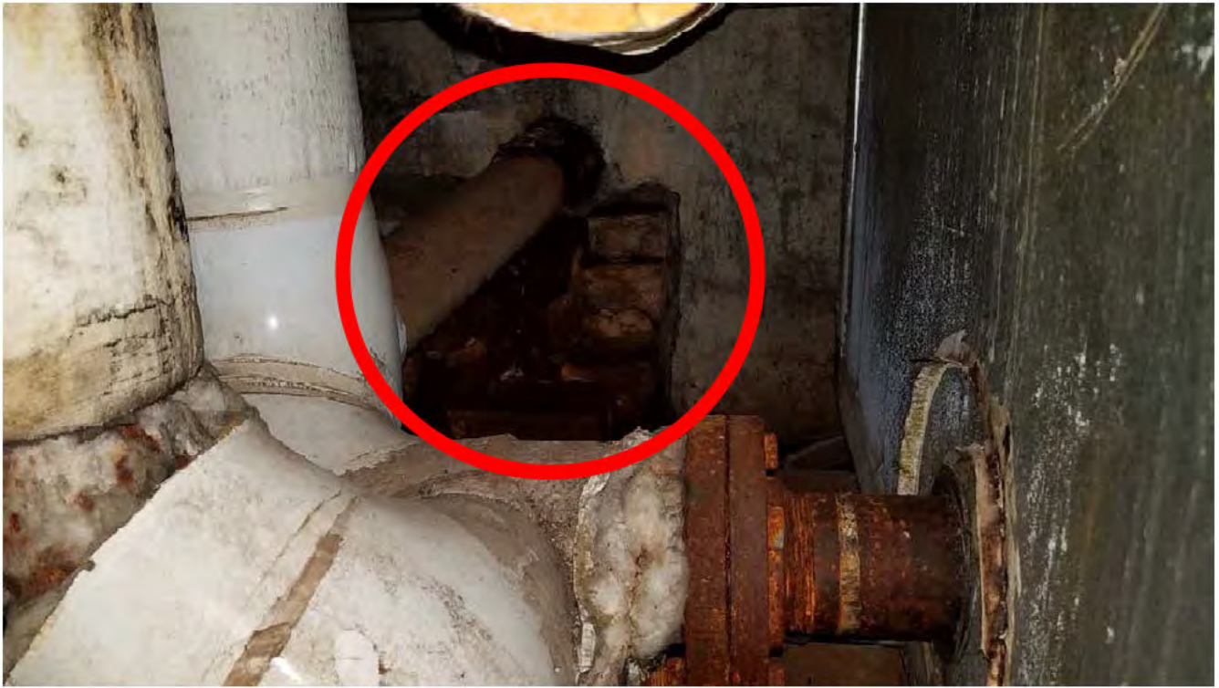
Water Leak Through Mechanical Room 2 Foundation Wall Pipe Penetration
