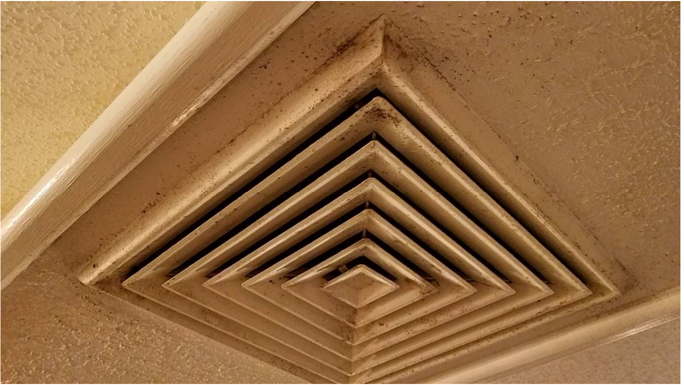
Lamplighter Dining Room Air Diffuser
