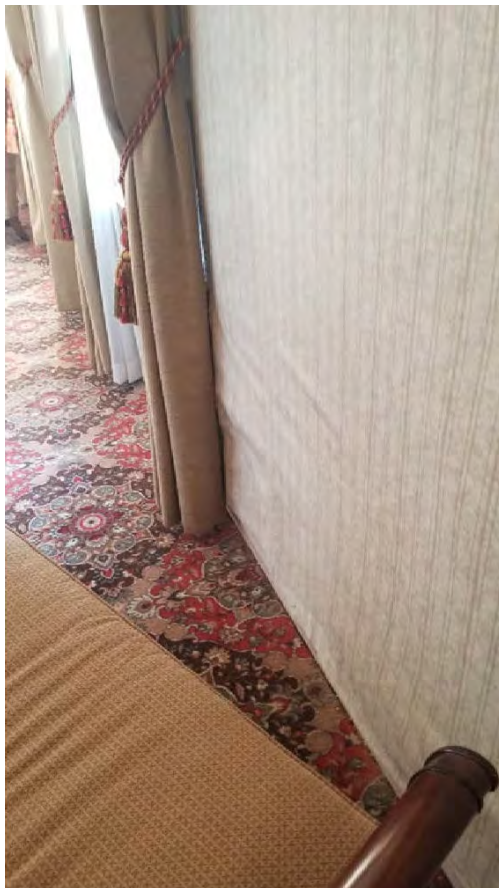
Water damaged wall behind textile
