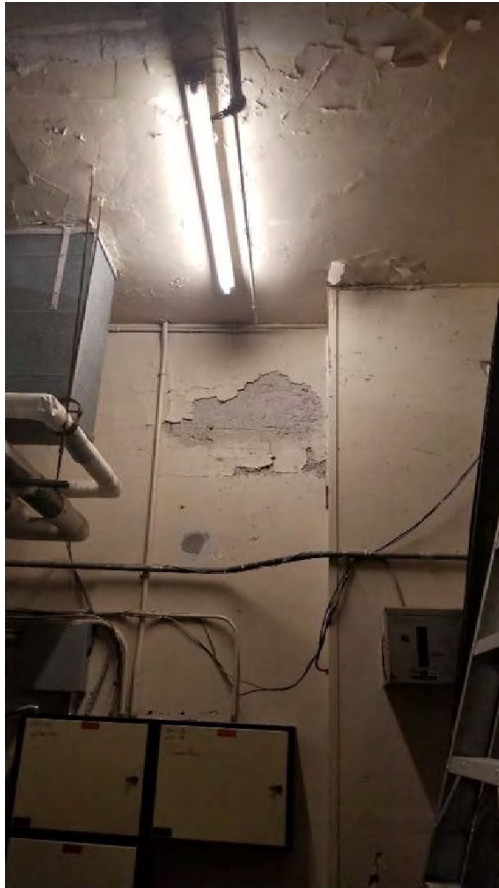
Ceiling/Wall water damage
