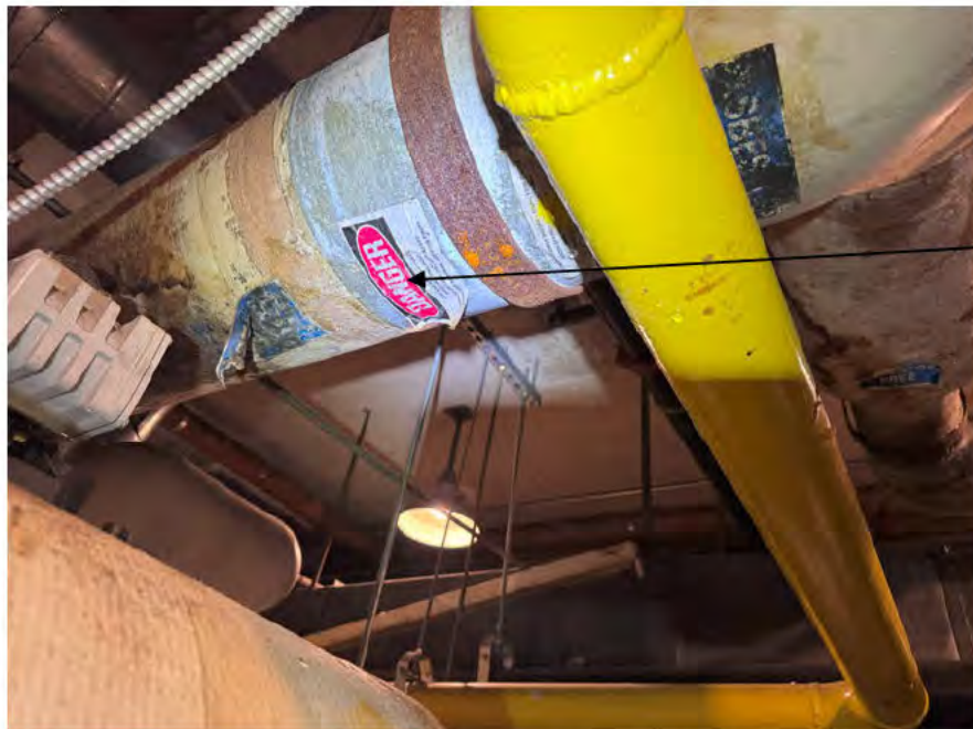
Photo 28: ACM pipe insulation observed in Basement Mech. Room 012.
