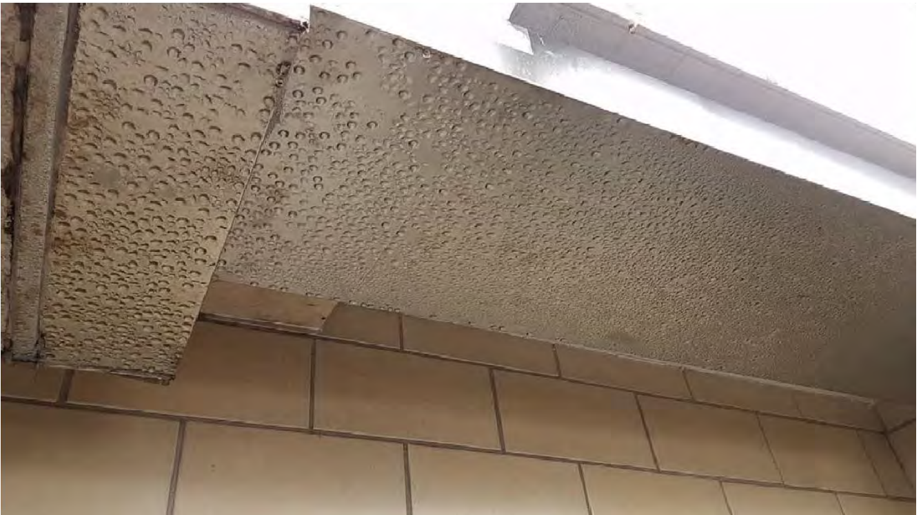
First Floor Kitchen Condensation on Dishwasher Duct – Inadequate Exhaust in Space
