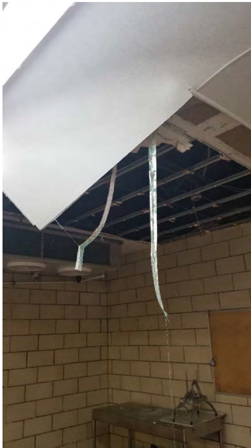
Ceiling water damage
