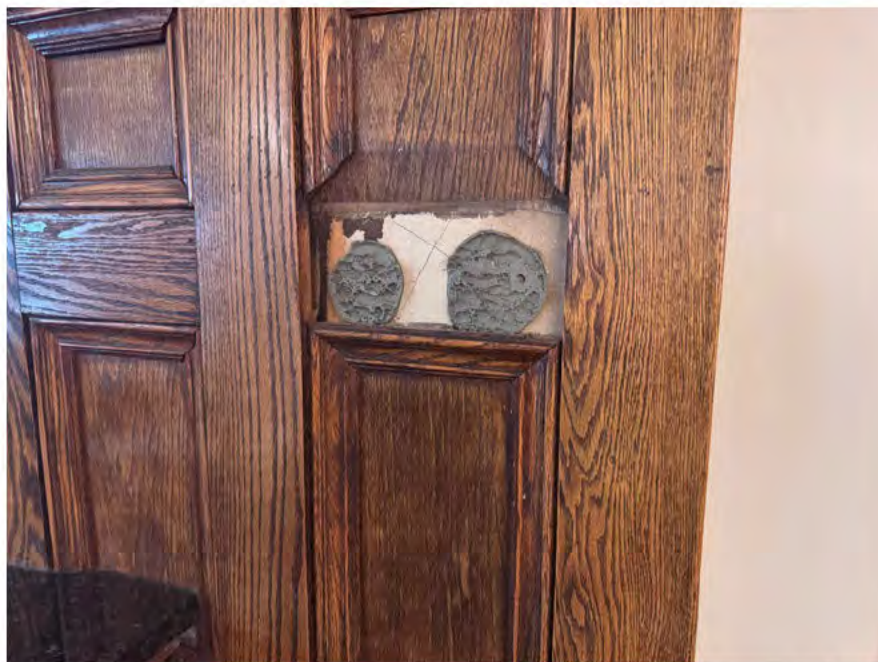
Photo 9: ACM brown adhesive pucks observed behind wood wainscoting in Dining Room 116 (Sample #61).
