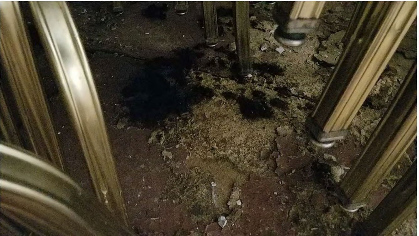
Coat Check Mechanical Room Mold Growth on Floor
