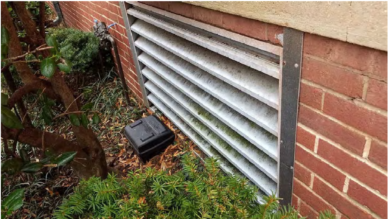
Outside Air Intake at Grade with Rat Trap In Front of It
