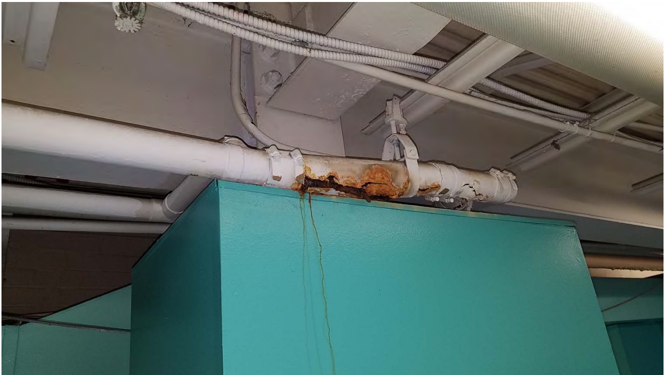
Bathroom Leaking Pipe
