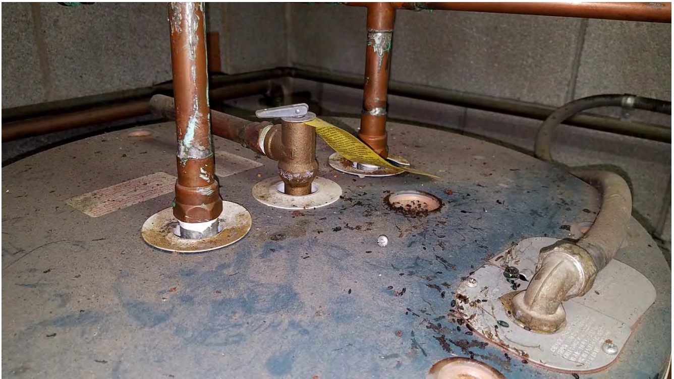
Bathhouse Women's Room Water Heater with Rodent Feces
