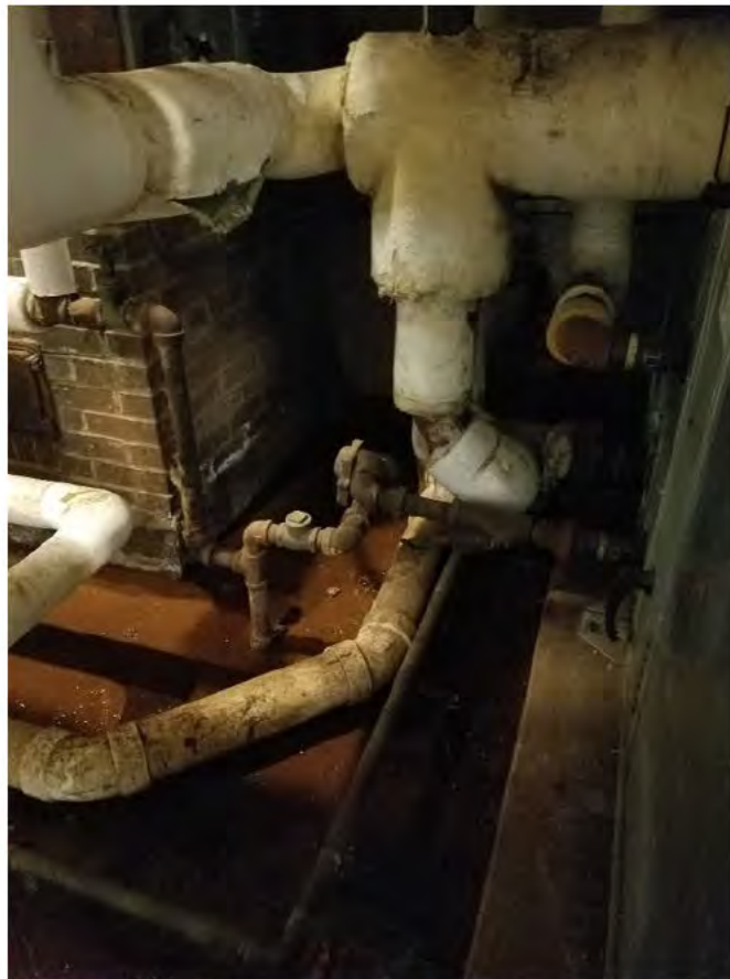
Water Leak Through Mechanical Room 2 Foundation Wall Pipe Penetration
