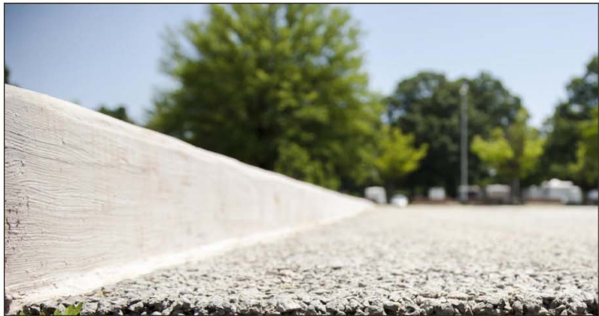
Shown is the permeable pavement across from the bioretention area. This shows the concrete layer of the permeable pavement that has cracks for water to pass through.
