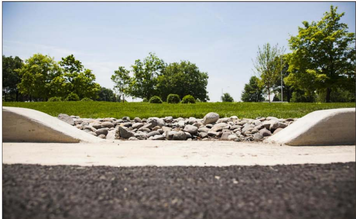
This is one of many parking lot inlets on the side of the bioretention area of the Stormwater BMP. Water drains into this inlet and is first filtered by stones before flowing into the grass and then down into the canal.
