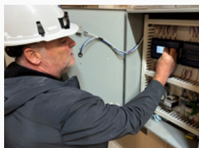
Patrick Rider, OMD, utilizes the direct digital control system to ensure optimal temperature, pressure and flow.
