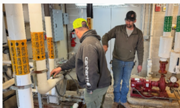
Garth Madere and Bill Hooper, Operations & Maintenance Division (OMD), work to address a leak at the heat exchanger of a mechanical room in the 87000 barracks block.
