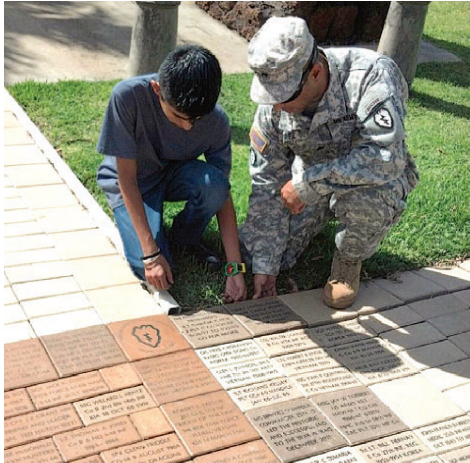
Staff Sgt. Carlos Ramirez Jr., headquarters commandant, Operations Co., HHBN, 25th ID, and his son, Carlos Ramirez III, lay new brick pavers at the 25th ID Headquarters to expand the courtyard adjacent to the "Unified Through Sacrifice Memorial," recently. (Photo courtesy 25th Infantry Division Public Affairs)
