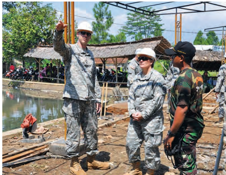
BOGOR, Indonesia — 1st Lt. Joseph Ruhnke (left), executive officer and commander, 871st Eng. Co., 411th Eng. Bn., 9th MSC, and 1st Lt. Nanang Sujarwanto (right), project operations staff engineer and officer in charge, Tentara Nasional Indonesia (Indonesian armed forces), meet with Brig. Gen. Michele Compton (center), former commander, 9th MSC, to discuss the status of a humanitarian civic action project as part of the 9th MSC's annual Garuda Shield exercise, here, recently. (Photo by Capt. Christina Douglas, 9th Mission Support Command)
