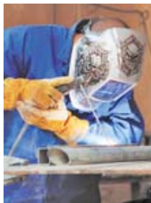
Spc. Raymond Ramos Fee, a welder with Forward Support Company, 65th Engineer Battalion, 130th Eng. Brigade, works on a welding project.
