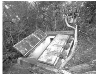
underground control station
