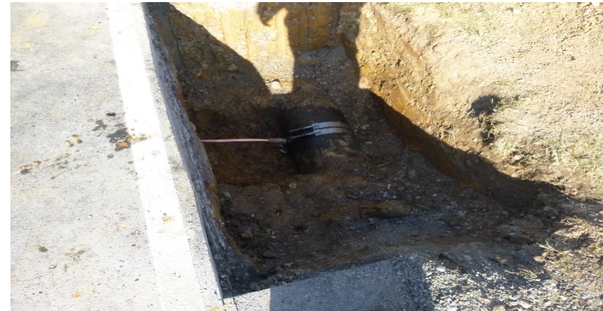
Water main saddle and service tap.
