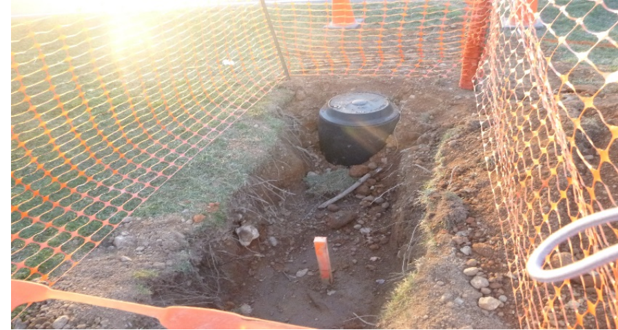
Water meter trench and associated housing.
