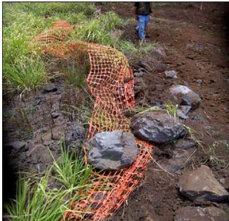
Photo 1: July 25, 2006 – Boulders rolled onto fencing
