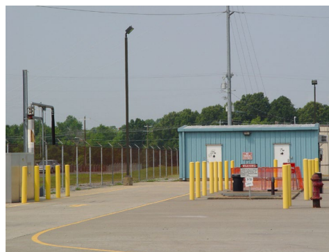
Oil Water Separator at BLDG 7085
