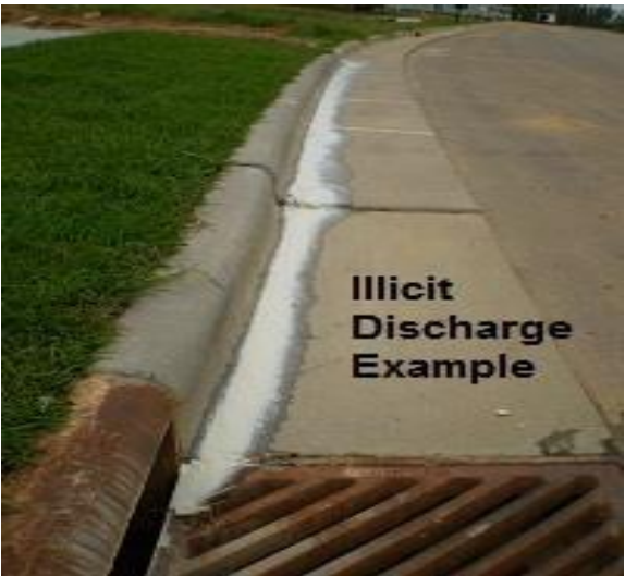
Potential outfall issue with presence of at least one physical indicator – paint stains
