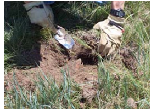
Fig 3. Excavating anomalies/sampling. explosive risk or other hazards. Soil sampling is necessary to determine if this risk exists (Fig 3).
