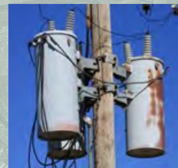
Typical PCB-containing Transformer
