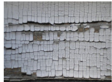
“Alligatored” lead paint
