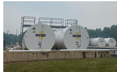
Aboveground Storage Tank
