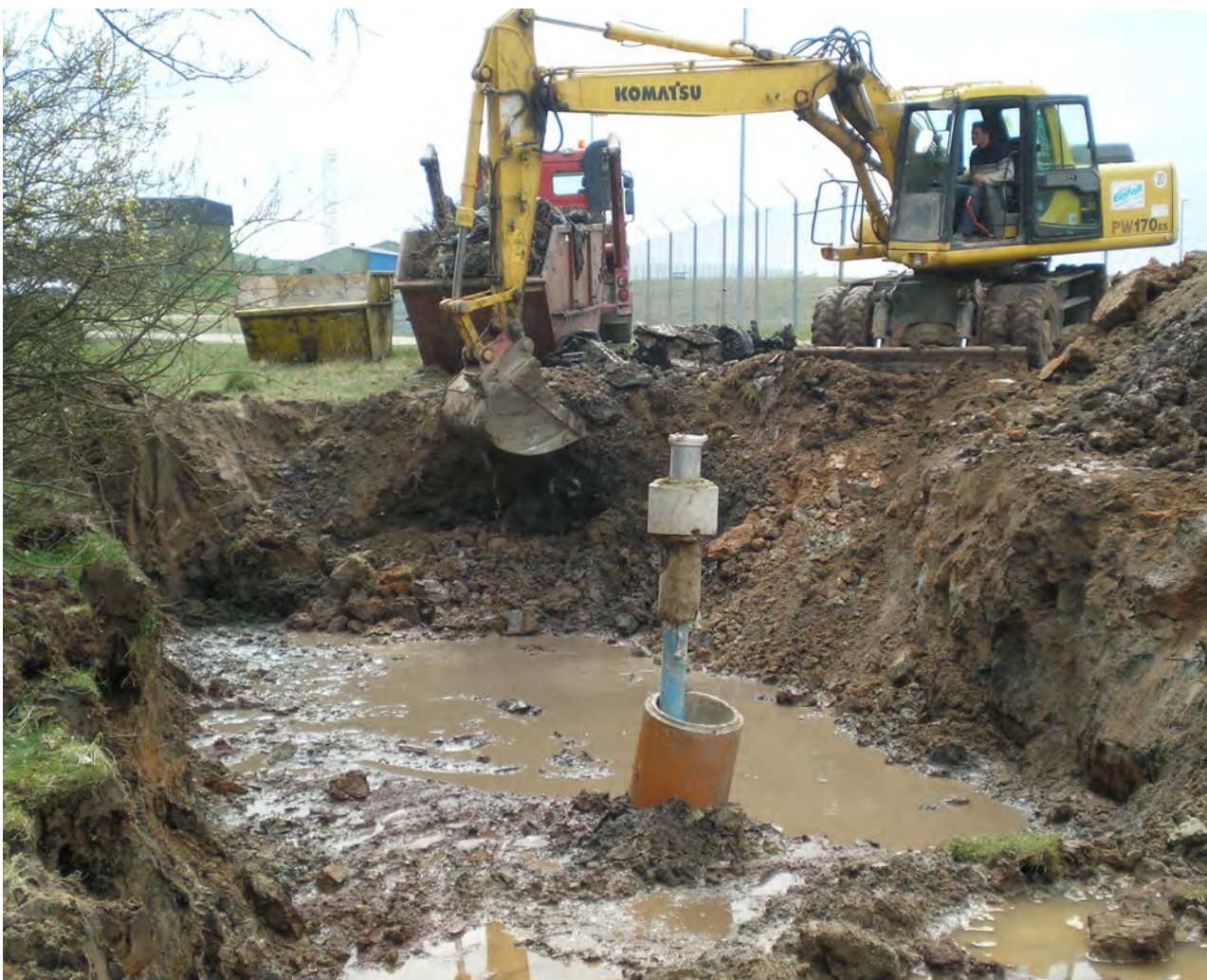
Excavation of contaminated soil and debris at a post-World War II landfill at Urtas, Ansbach.
